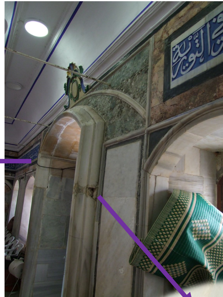
Damage to the lintel Above the entranceway
